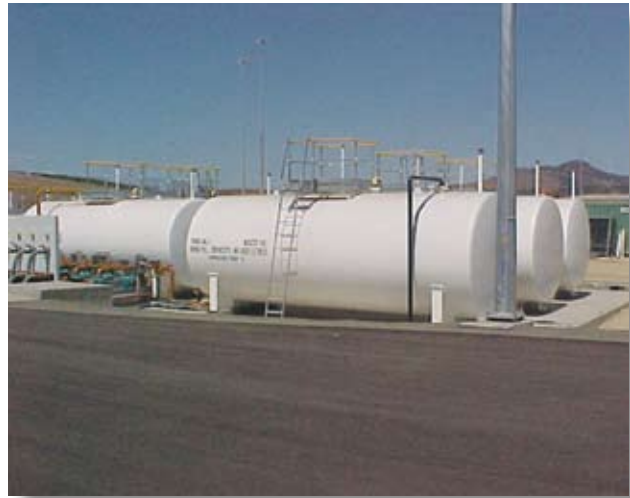
Fuel Tank Farm
