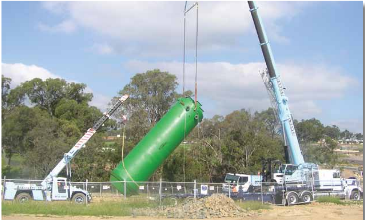
Mullaly FRP Lift Station – 2.750 Diameter x 10.600 Deep
