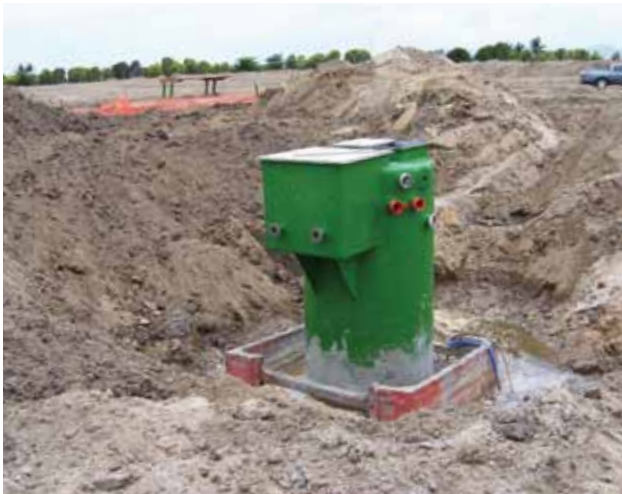
Mullaly FRP Combo Pump Station 2.750 diameter x 6.700 deep (High Water Table Installation)
