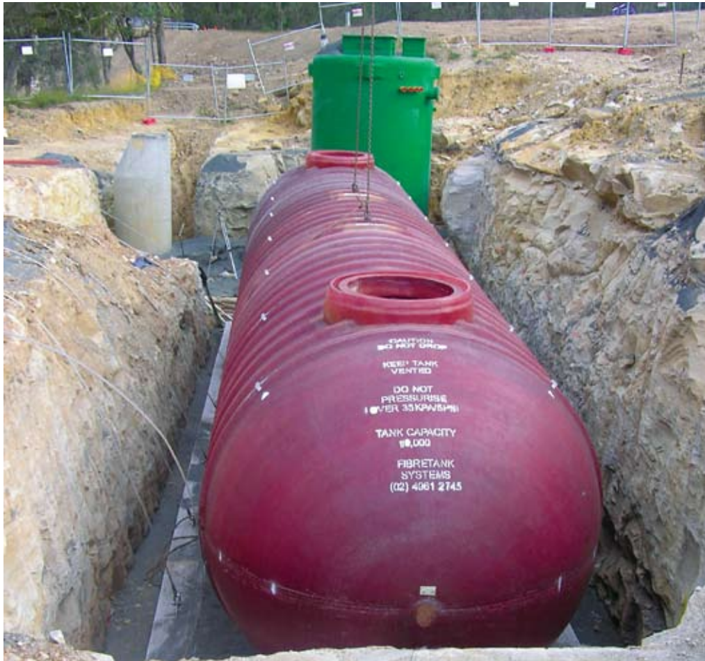
110,000 litre Sewage Tank
