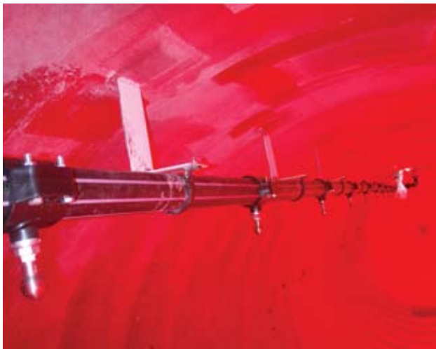
Sewage Tank Cleaning System
